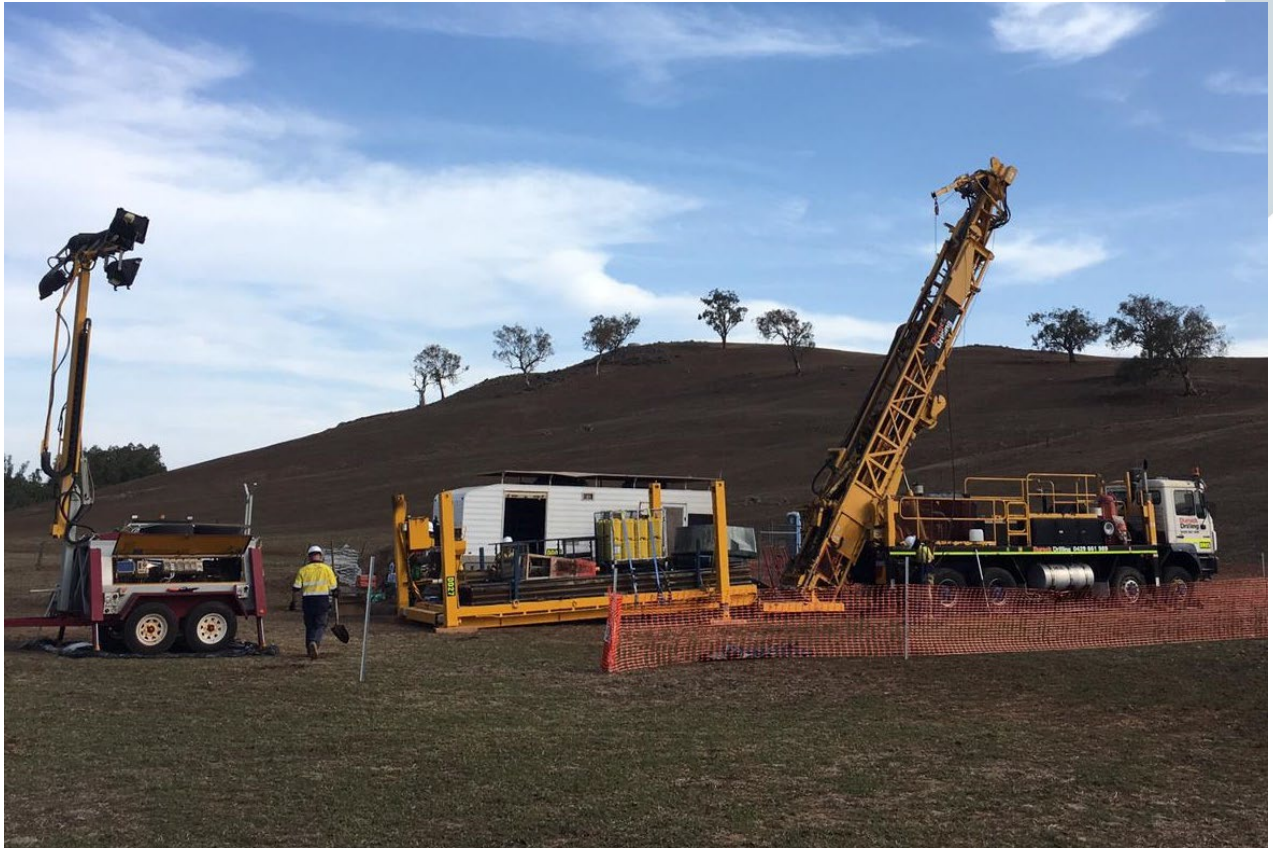
Figure 5: Diamond drill rig mobilised on site at the Junee Copper-Gold Project, NSW.
